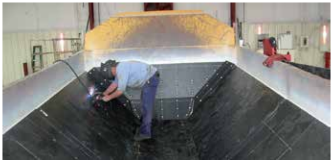
Strongly anchored: Installation of Matrox sheets in a funnel-shaped dump truck using the stud-welding process.
