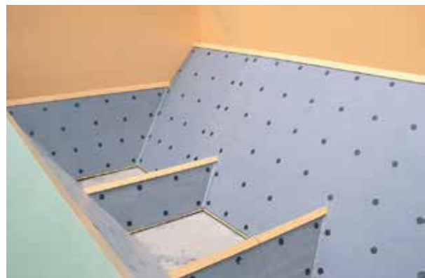
Hopper lining with weld stud, nuts & plugs. The distribution of fixing points can be clearly seen.
